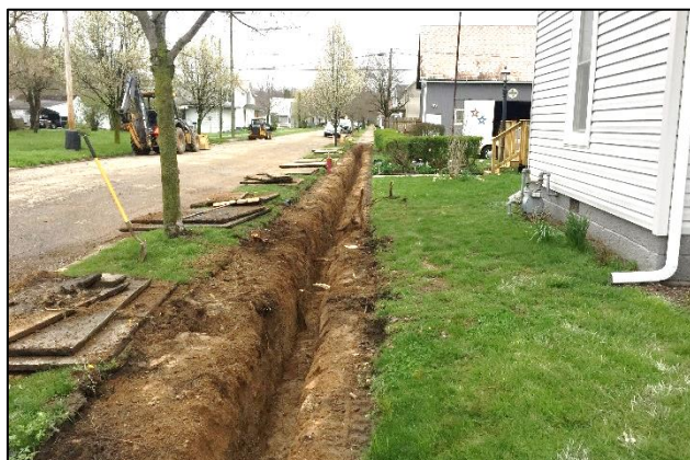
Trench excavated along the east side of Oak Street for installation of a new Columbia Gas main line. A new concrete sidewalk will be provided.
