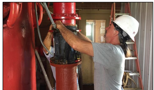
Doll-Layman, Ltd. is the project contractor. Doll-Layman workers are shown here making improvements to water lines inside the plant.
