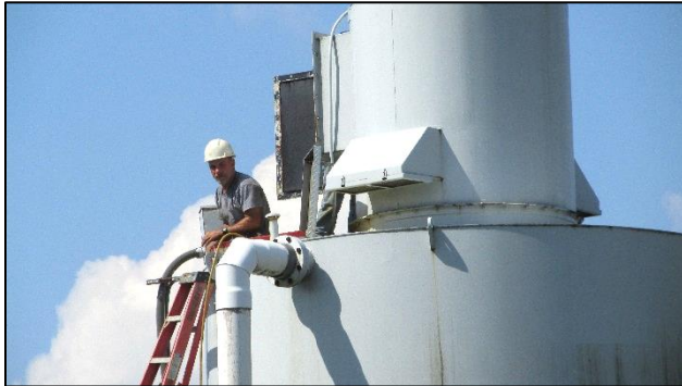
Doll-Layman, Ltd. employee preparing to clean and make repairs to the holding tank interior.
